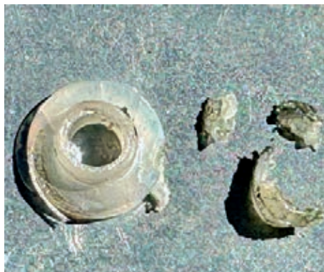
The remains of the original top hat insulation washer.
